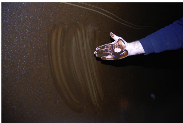
Fig. 2. Photograph from inside trunk main showing material adhesion across all boundary surfaces.
