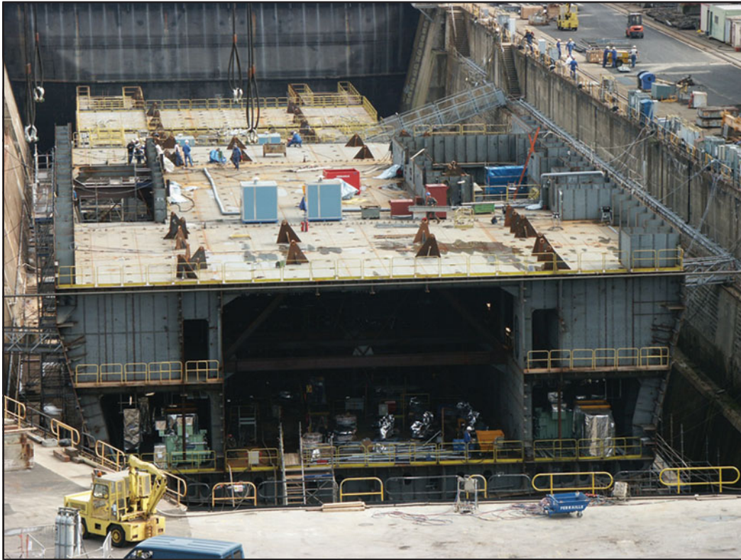
Figure G.2 Building of the Rear Section of the Mistral by Direction des Constructions Navales in Brest, September 2003
