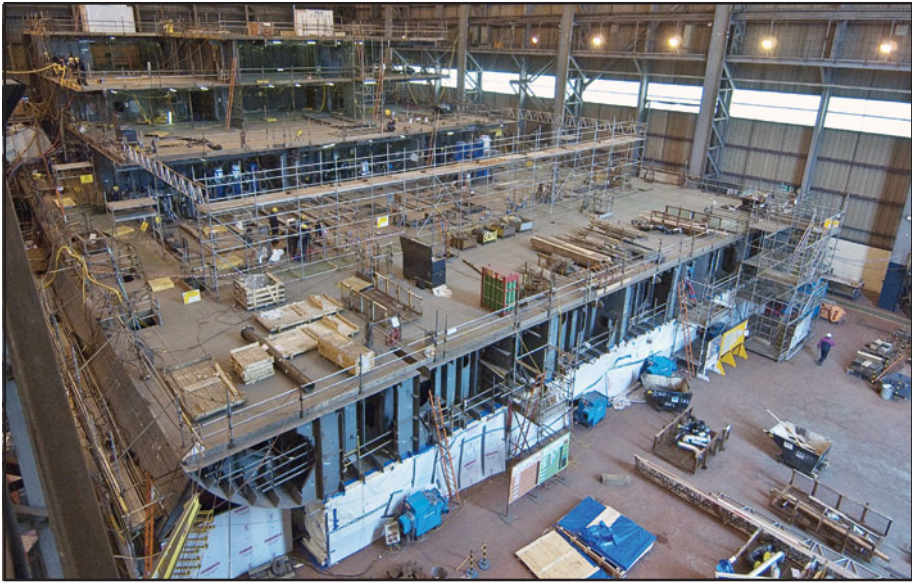
Figure F.3 Early Stages of Construction of HMS Queen Elizabeth Lower Block 3 at BAE Systems Surface Ships Govan Shipyard
