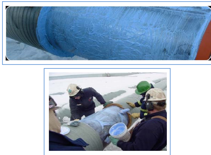
Figure 12: "above the Arctic circle" application: corrosion under insulation.
