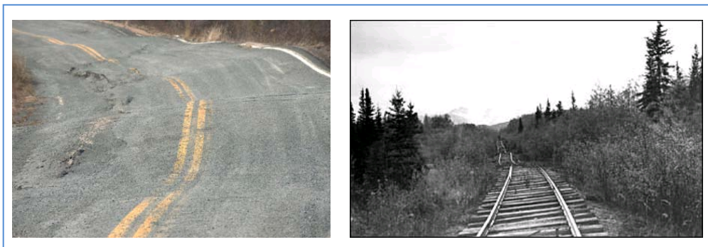
Figure 4: Thawing permafrost under roads and railway tracks
