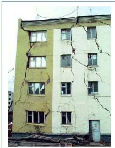
Figure 3: How thawing permafrost can destroy a building (Chersky, Russia) ( www.klimanotizen.de )
