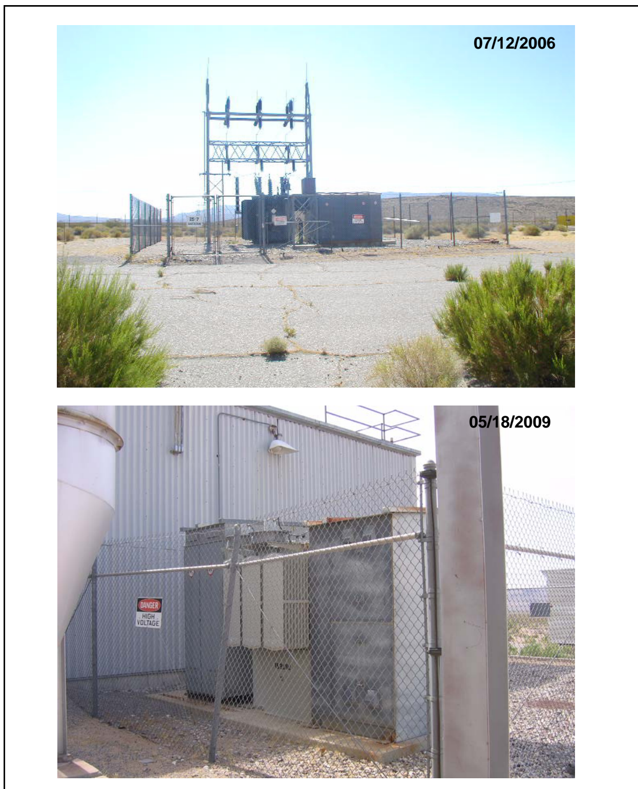
Figure 2-4 Substations Southeast (top) and Southwest (bottom) of Building 3900
