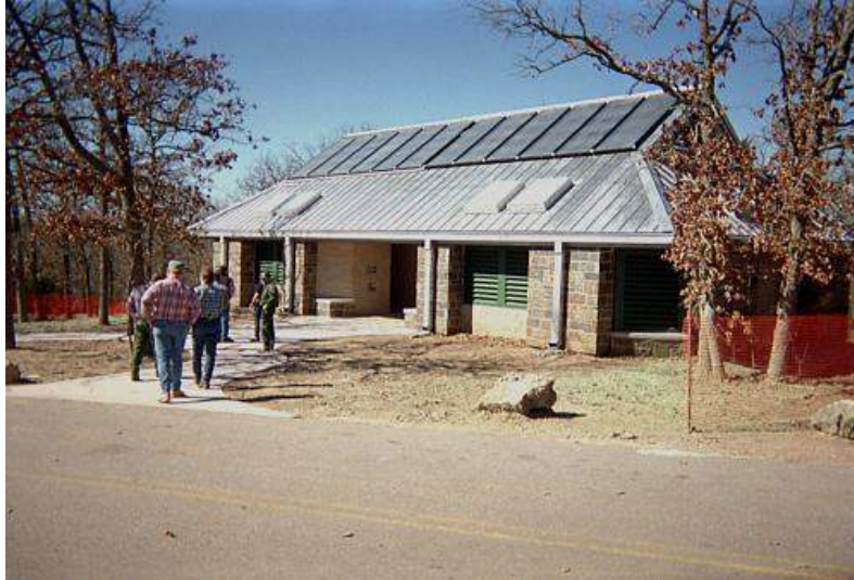
Figure 5. Flat plate (boxed) solar domestic hot water heating system for showers and laundry at Chickasaw National Recreation Area in Oklahoma. Credit: Andy Walker, NREL
