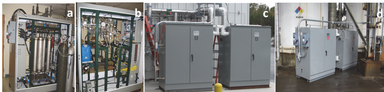
Figure 2. TDA's field demonstration unit; (a) the 4-bed high temperature PSA-based CO 2 separation sub-assembly; (b) synthesis gas conditioning sub-assembly, (c) TDA's field demonstration unit installed at the Power Systems Demonstration Facility, (d) TDA's field demonstration unit installed at the Wabash River IGCC power Plant.
