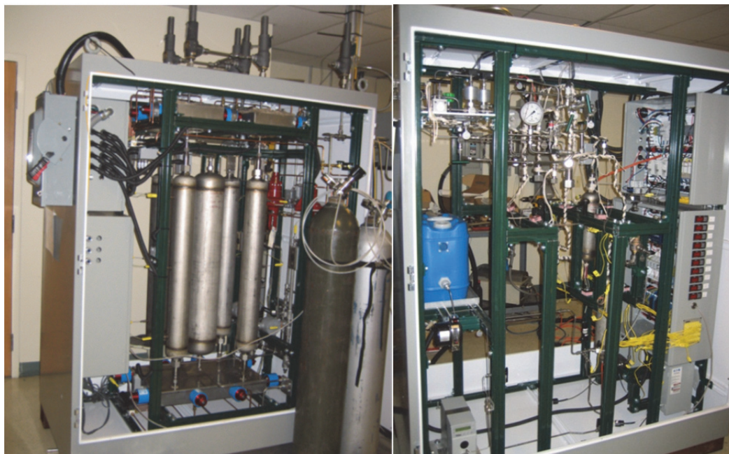
Figure 72. CO 2 Adsorption Unit (Left) Gas Conditioning Unit (Right) inside NEMA enclosures.
