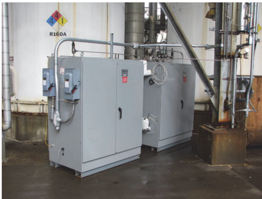
Figure 86. Test Unit installed at the Wabash River IGCC Power Plant.
