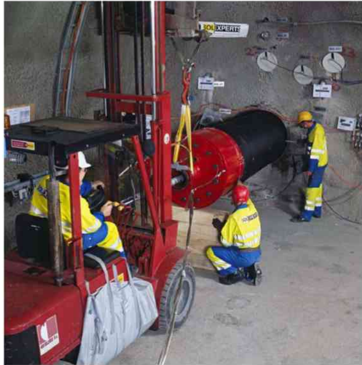
Figure 3-26. HG-A Experiment at Mont Terri URL: Installation of packer system (from Marschall et al., 2012).
