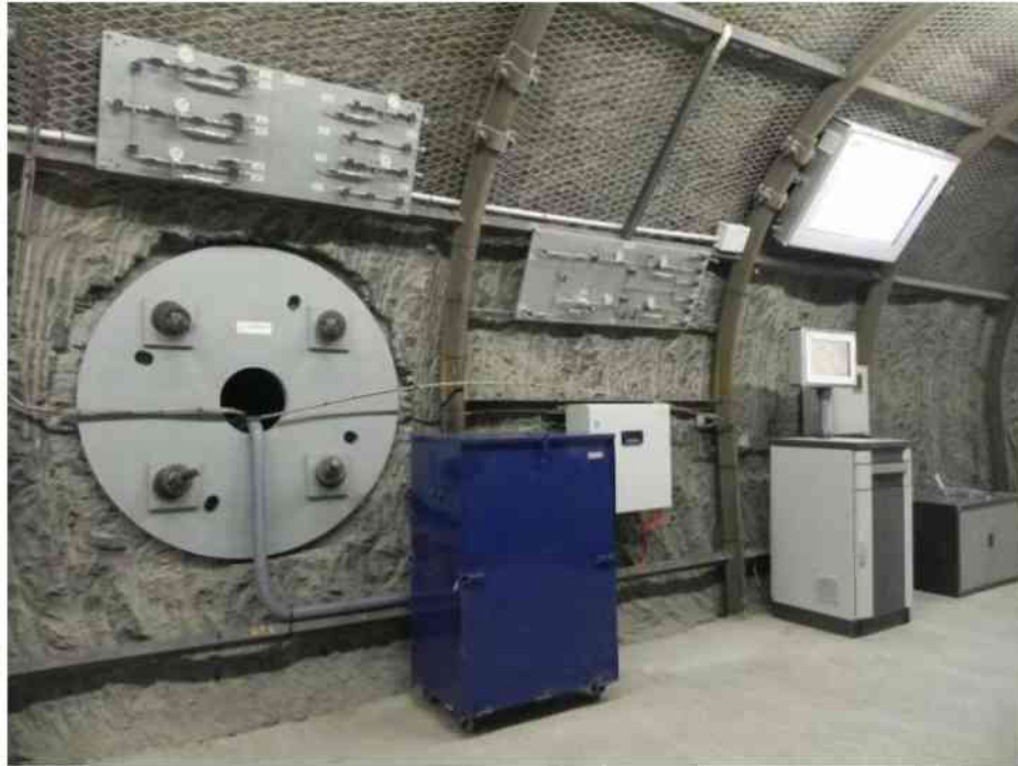
Figure 3-3. SEALEX Experiment at the Tournemire URL: View of mini-tunnel from gallery after core emplacement (from Barnichon, 2011)
