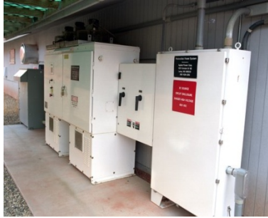
Figure 5. String inverter. Photo by Warren Gretz, NREL 07985
