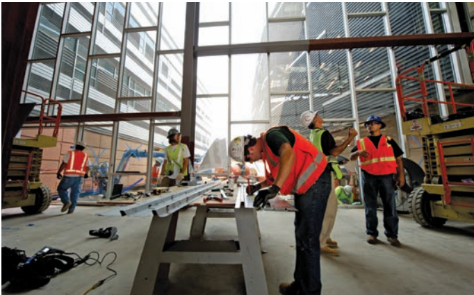
NREL's Energy Systems Integration Facility during construction. Photo by Dennis Schroeder, NREL 22119
