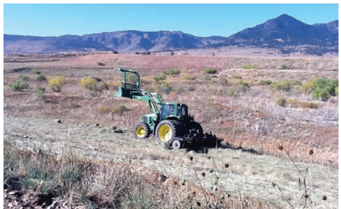
Reseeding and mulching following construction activity at NWTC. Photo by Genny Braus, NREL 24489
