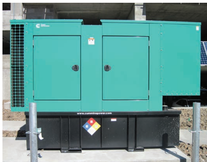
New standby electrical generator and AST at the STM parking garage. Photo by Larry Durbin, NREL 24487
