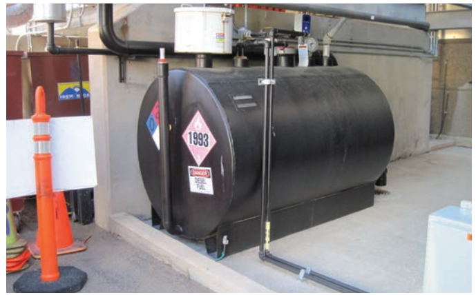
Diesel storage tank at the STM site. Photo by Larry Durbin, NREL 24478
