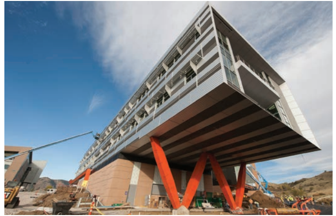
Construction of the new Energy Systems Integration Facility. Photo by Dennis Schroeder, NREL 22670
