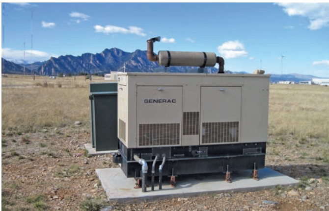
Standby electrical generator at the NWTC. Photo by Larry Durbin, NREL 24490
