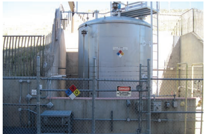
A 6,000-gallon ethanol tank at the IBRF on the STM campus. Photo by Larry Durbin, NREL 24477
