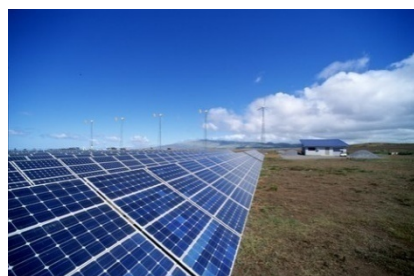
Source: NREL PIX 13823
