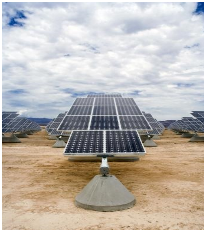
Source: NREL PIX 15280
