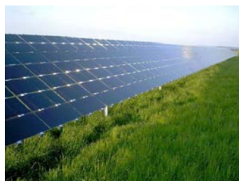
Source: NREL PIX 14726
