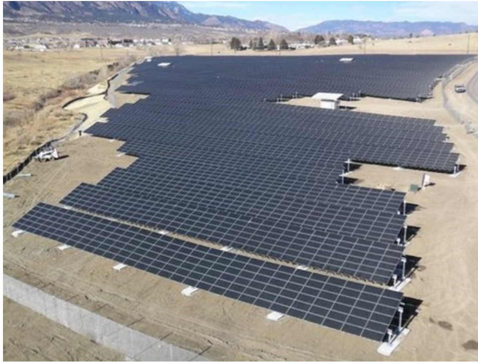
Source: NREL PIX 17394
