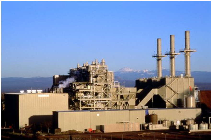
Figure 3. Direct-fired biopower system. Photo by Wheelabrator Shasta Energy Co., NREL 07163
