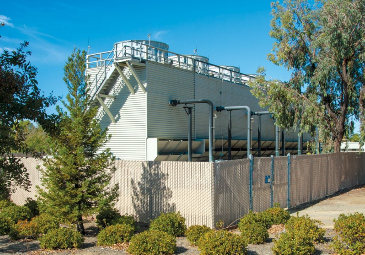
Cooling towers, which feed water to the air-conditioning systems for the Laboratory's high-performance computing facilities, account for about 45 percent of the total water consumption at Livermore's main site. (Photograph by Lee Baker.)
