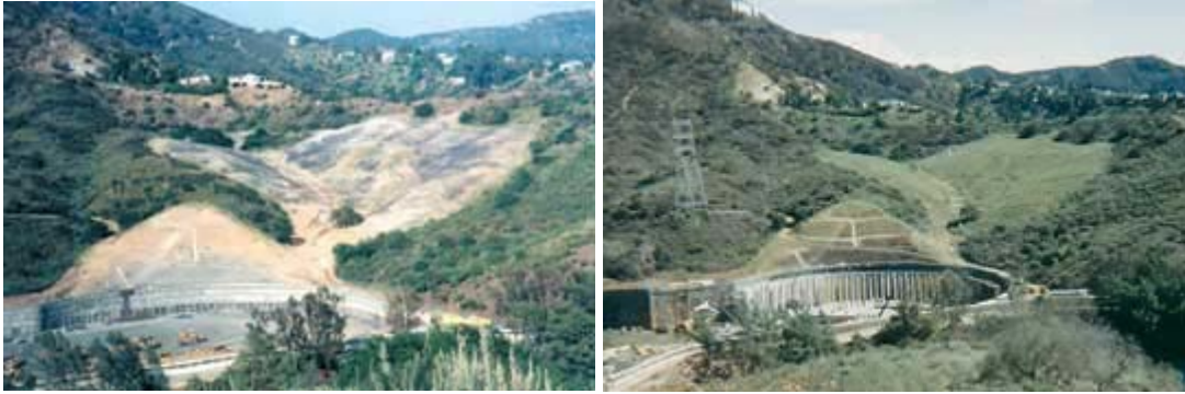
Figure 7. An example of successful revegetation on a canyon fill project where soils were compacted to 90 percent. The left photo is after grading and the right photo, after an intense rain event, shows how the stabilization and revegetation efforts protected the project area from water erosion (photos of Hollywood Hills, California, from Gray, 2002).
