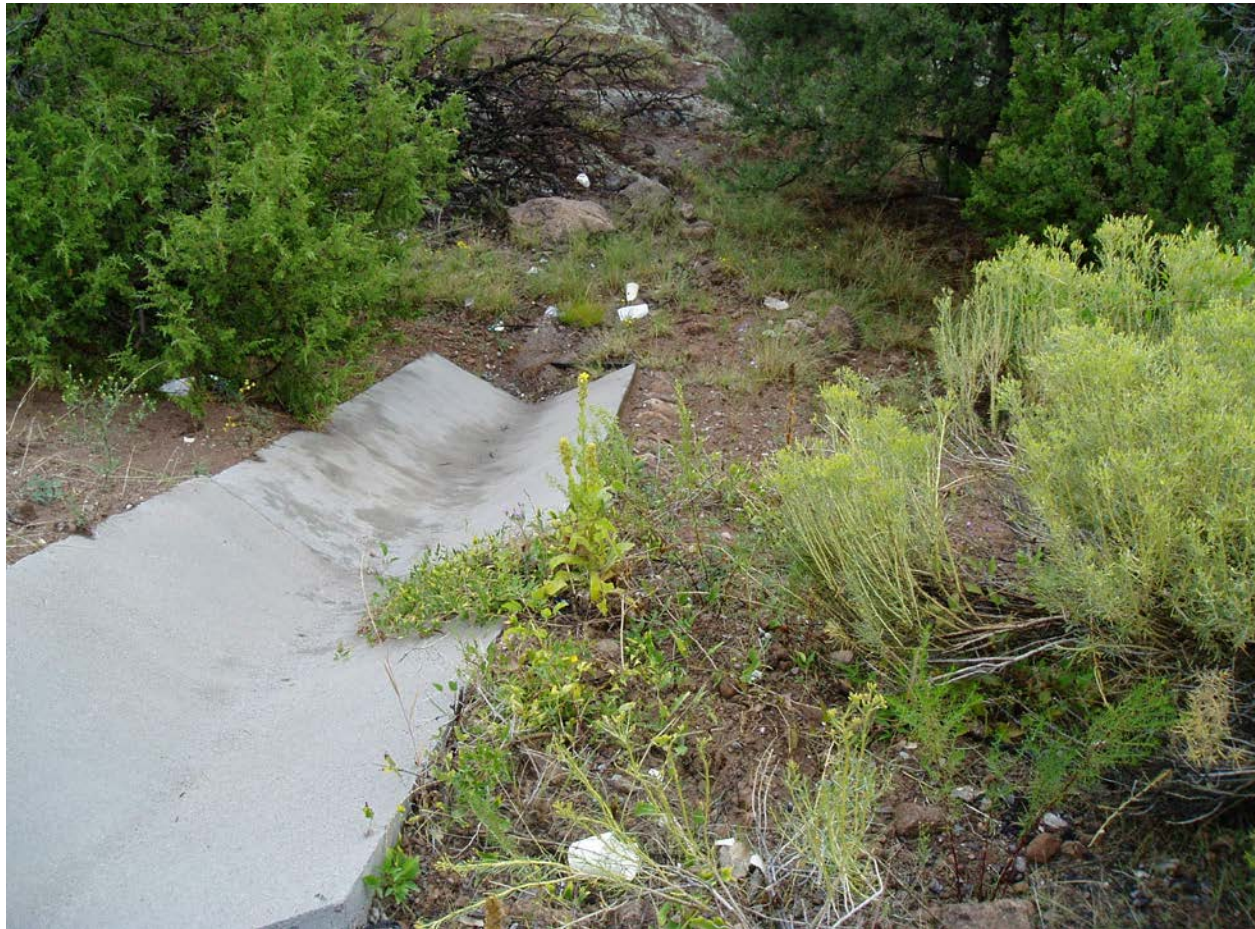
Garbage at the bottom of the swale
