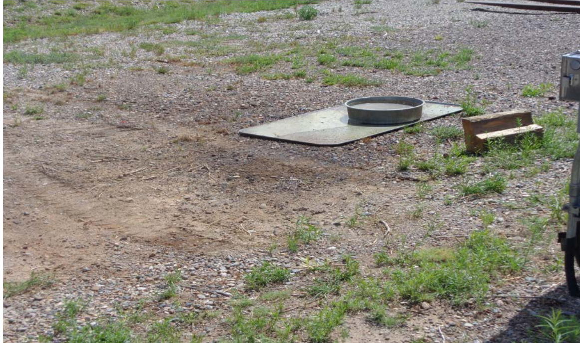
Stained base course and Spill pans containing free liquids
