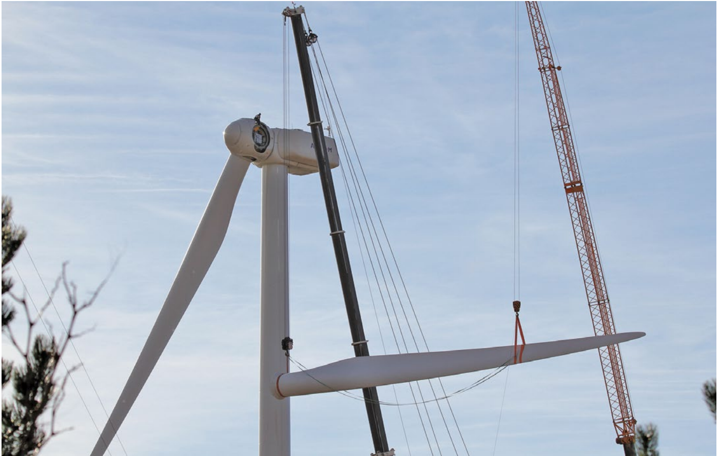
New blades are being installed for testing on a 3MW wind turbine at NREL's National Wind Technology Center. Photo by Lee Jay Fingersh, NREL 33210
