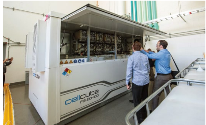
Energy Systems Integration Facility researchers inspect the vanadium redox flow energy storage system, which is being tested to assess its ability to provide uninterrupted power supply from renewable energy sources. Photo by Dennis Schroeder, NREL 31367
