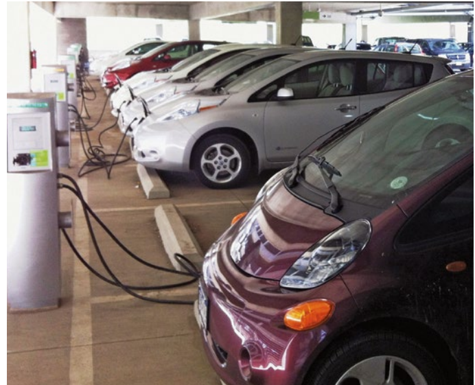
Electric vehicle charging stations at the STM campus parking garage. The 36 charging stations are part of a research project to test the impact of charging scenarios on the electrical distribution network. Use of electric cars has the potential to reduce carbon dioxide emissions that contribute to climate change. Photo by Erik Nelsen, NREL 26488
