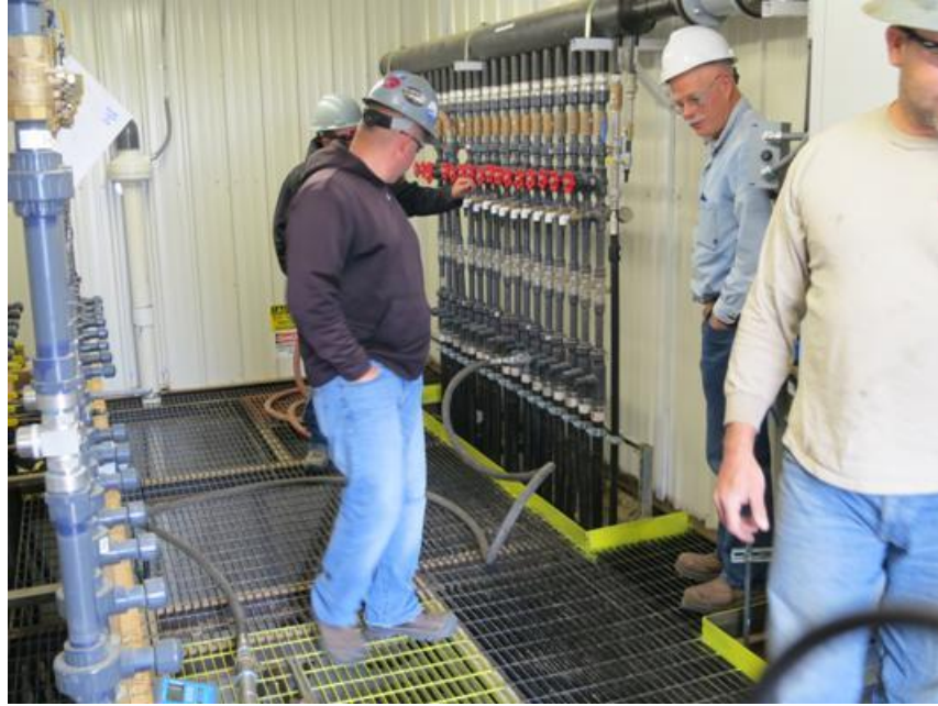
Figure B-5. Injecting MP-423 water into 7P-30 at Header House 7-5.
