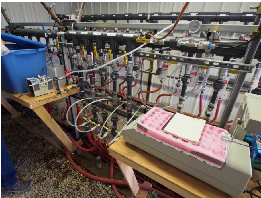
Figure A-4. Close-up view of circulation loop plumbing for 4P-121 well pattern.
