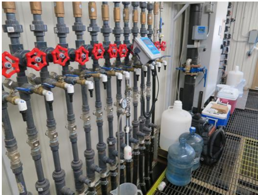
Figure B-8. Plumbing on production wellhead to divert flow to autosamplers and YSI flow cell. Sample collection point for filtered grab samples for uranium isotope analyses is shown.
