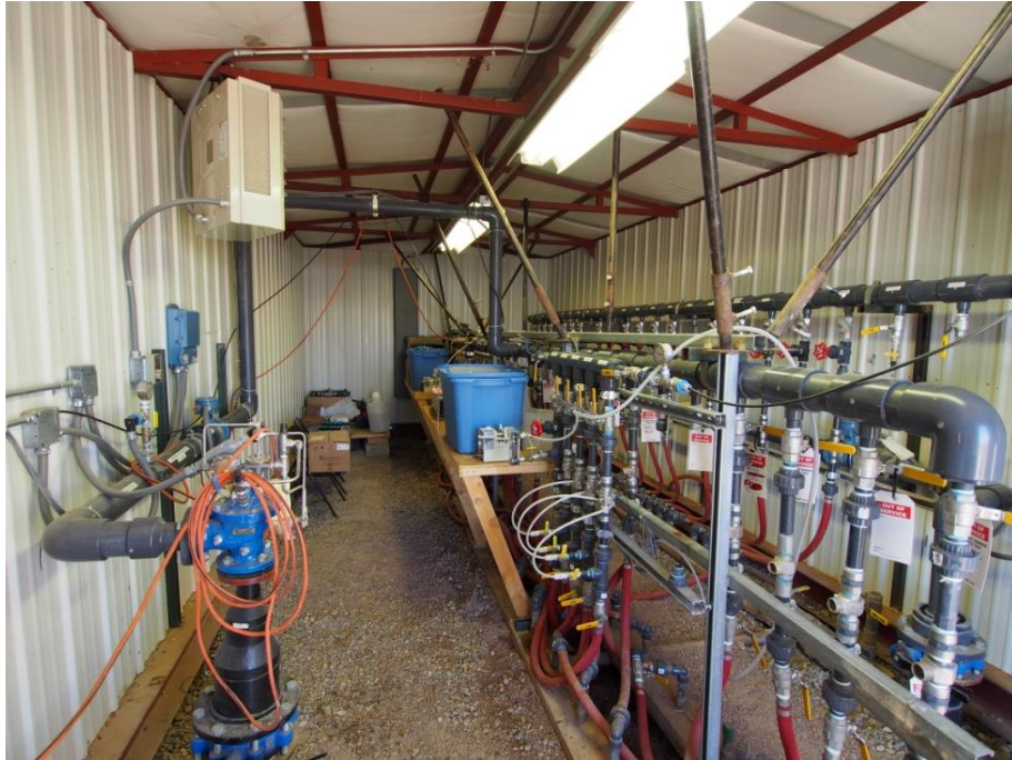
Figure A-3. View inside Header House 4-6 during cross-well tracer test.
