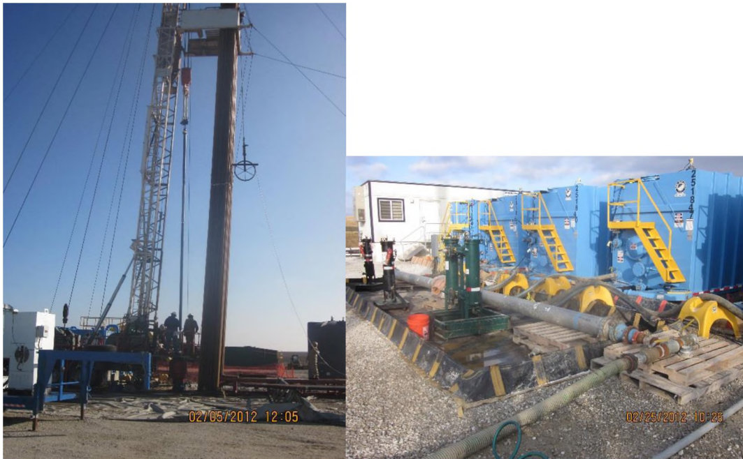
Figure 4.29. Installing the Submersible Pump (left); Water Storage Tanks (right)
