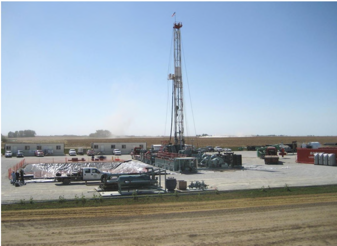
Figure 4.25. Stratigraphic Borehole FGA-1 Drilling Location (looking south). Lined earthen pit is visible in foreground.
