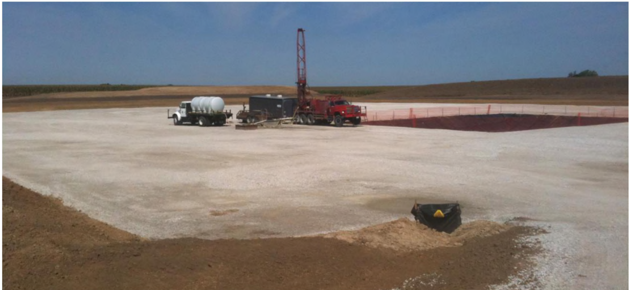
Figure 4.20. The FutureGen 2.0 CO 2 Storage Site Shallow Borehole Being Drilled Using a Mud-Rotary Rig. Fenced-off area to the right is the reserve mud pit for stratigraphic well FGA-1.
