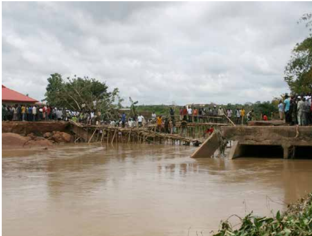
Collapsed bridge linking Apete to other parts of Ibadan, 2011
