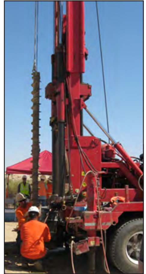
Figure 9. Test-drilling by consultants for Pacific Gas and Electric to install monitoring wells for flow-path studies, Hinkley, California, August 2015.
