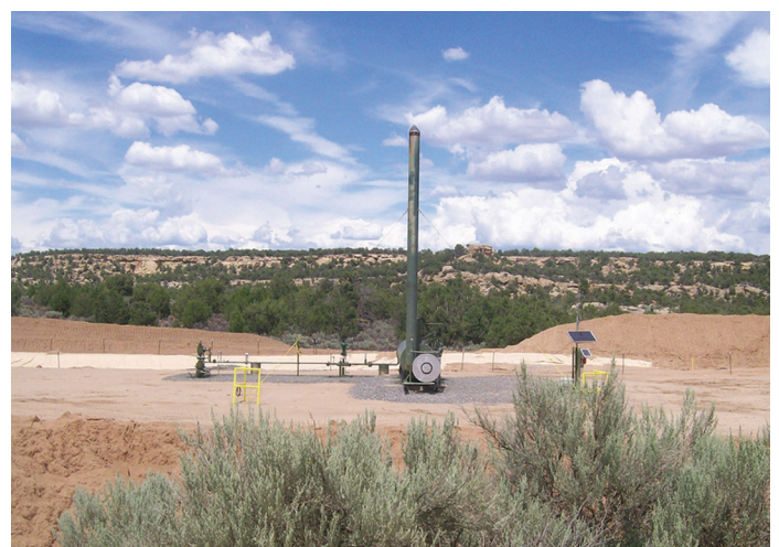
Figure 3. CO 2 injection well at the Pump Canyon test site in New Mexico. The well was drilled by the Southwest Regional Partnership on Carbon Sequestration (sponsored by the U.S. Department of Energy) to test the effectiveness of storing CO 2 in deep, unminable coal seams (Koperna and others, 2009). Similar wells could inject CO 2 for storage in depleted oil and gas reservoirs. Photograph by Eelco Kruizinga; used with permission.
