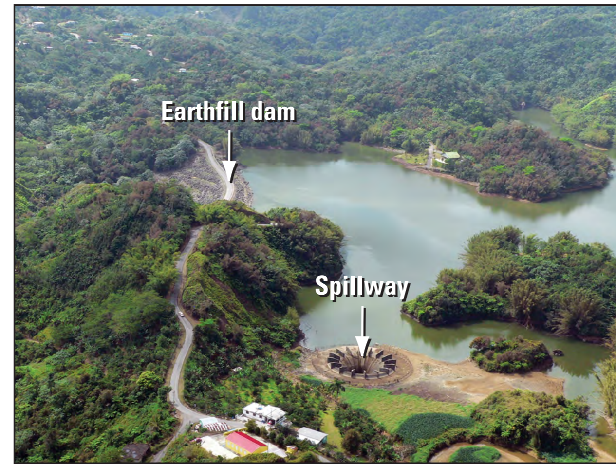
Figure 2. Aerial photograph of the Lago Garzas earthfill dam and spillway section, taken during a dam safety inspection in May 2006. Photograph courtesy of the Puerto Rico Electric Power Authority.
