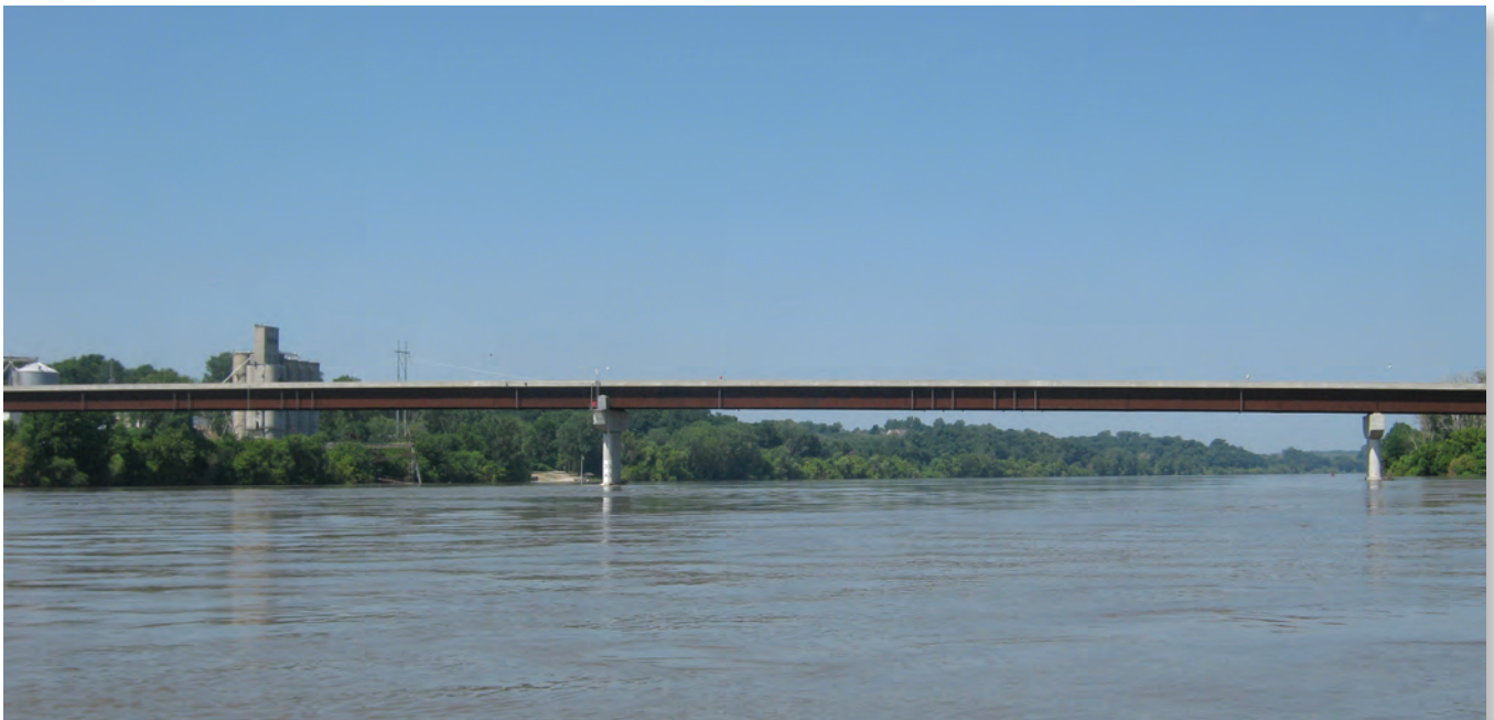
Structure A5910 on U.S. Highway 24 at Waverly, Missouri. Photograph by Joseph Richards, USGS.
