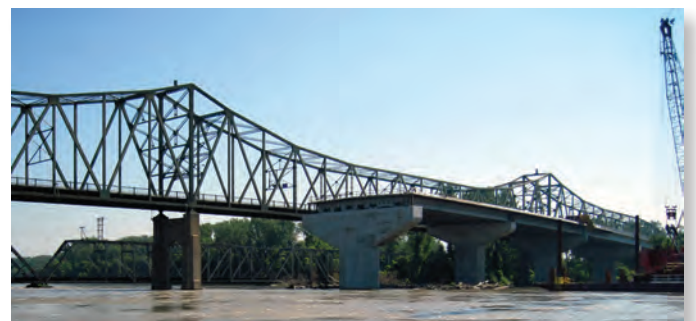
Structure 59-3-16.38 (013) on U.S. Highway 59 at Atchison, Kansas. The new U.S. Highway 59 bridge is being constructed in the foreground, and the Atchison railroad bridge is in the background.
