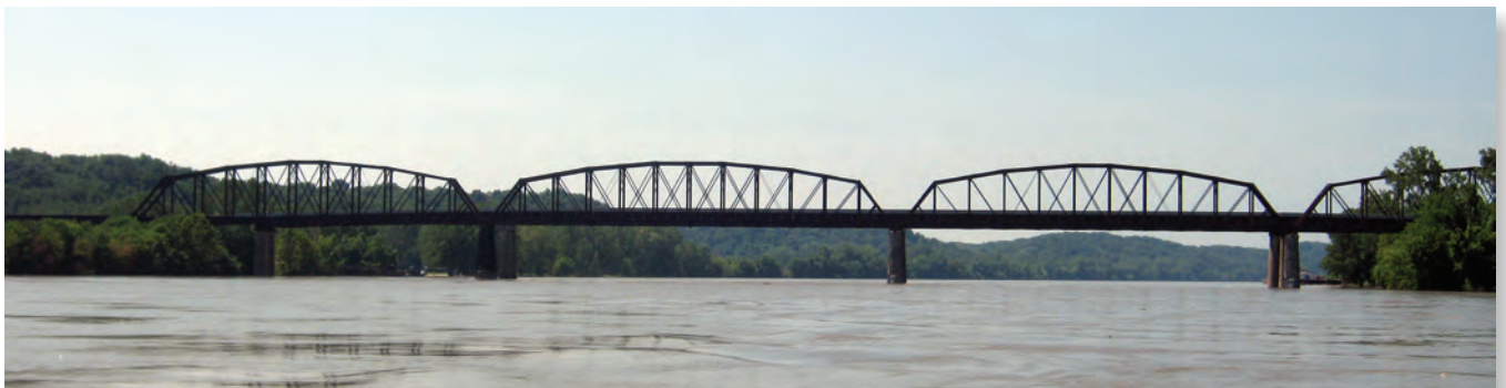
Structure G0069 on State Highway 240 at Glasgow, Missouri. The Glasgow railroad bridge is in the foreground. Photograph by Joseph Richards, USGS.
