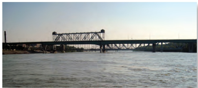
Structure A4060 on State Highway 9 in Kansas City, Missouri. The Armour-Swift-Burlington railroad bridge is in the immediate background.
