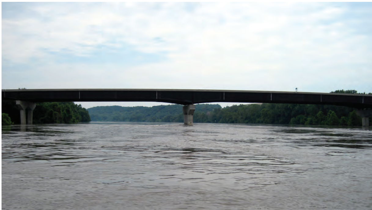
Structures 435-105-11.97 (235) and 435-105-11.98 (240) on Interstate 435 near Kansas City, Missouri. Structure 435-105-11.98 (240) is in the foreground and structure 435-105-11.97 (235) is in the background.
