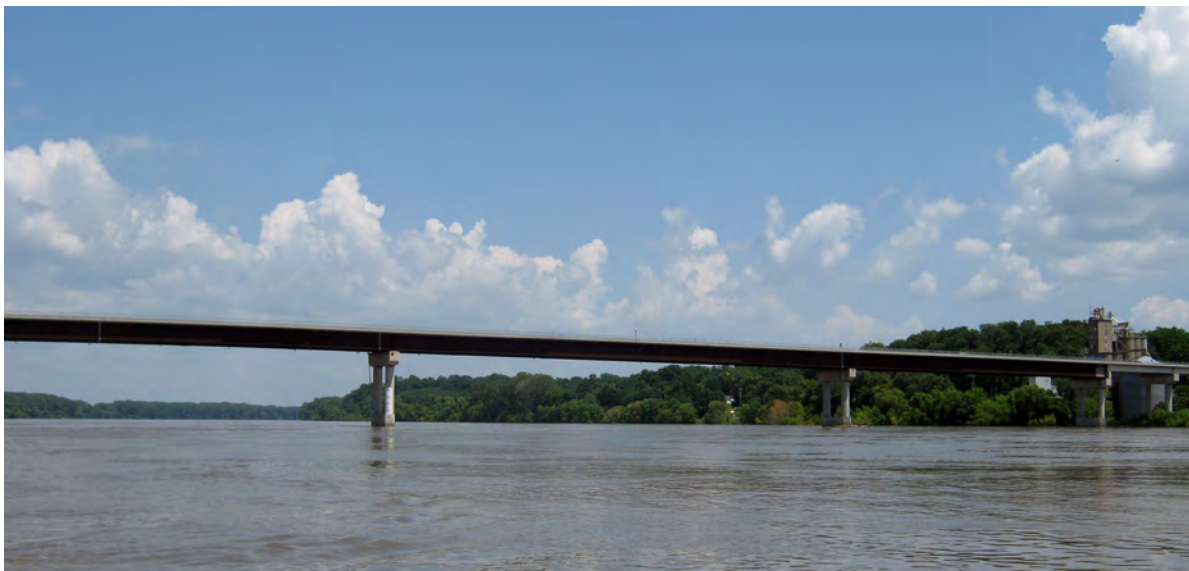
Structure A4574 on State Highway 5 at Boonville, Missouri. Photograph by Joseph Richards, USGS.
