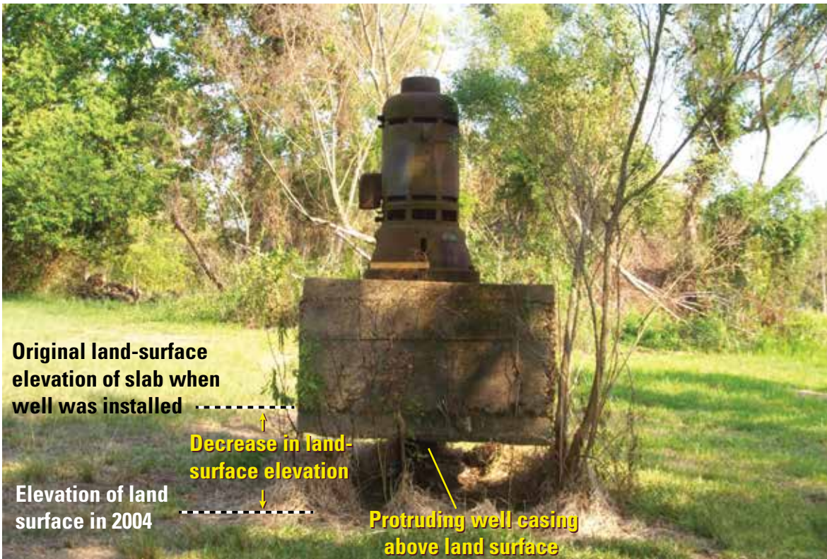
Figure 2. Damaged water well with the lower section of slab and well casing protruding above land surface because of a decrease in land-surface elevation in Baytown, Texas, September 2004.
