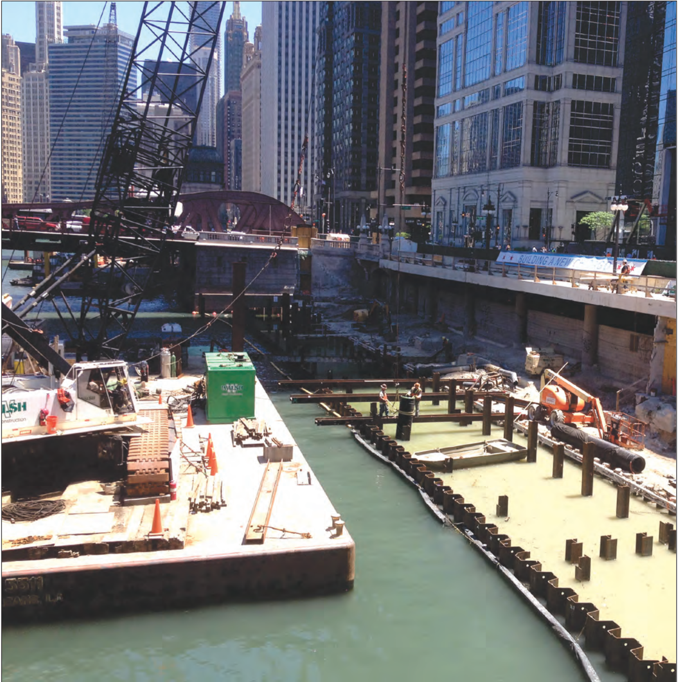
Figure 36. Construction of the river walk along the mainstem of the Chicago River.
