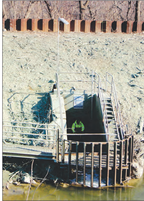
Figure 26. The entrance to the Summit Conduit and the location of the streamflow-gaging station.
