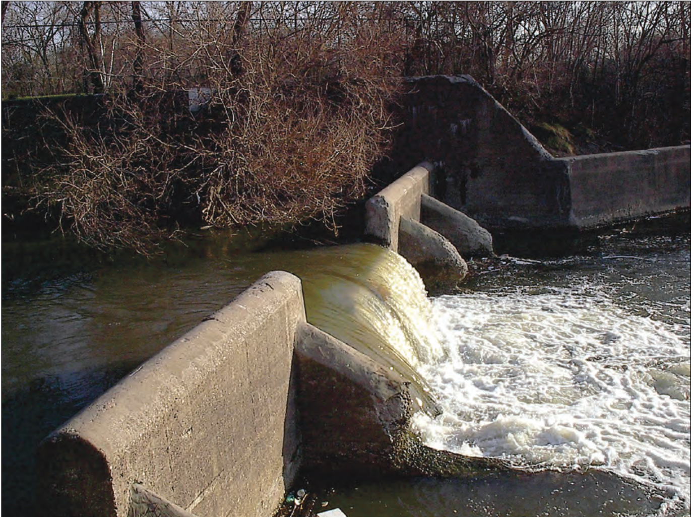
Figure 14. The concrete control structure at the confluence of the North Branch Chicago River and the North Shore Channel, Chicago, Illinois, and vicinity. (Photograph by Shawn Cutshaw, U.S. Geological Survey)
