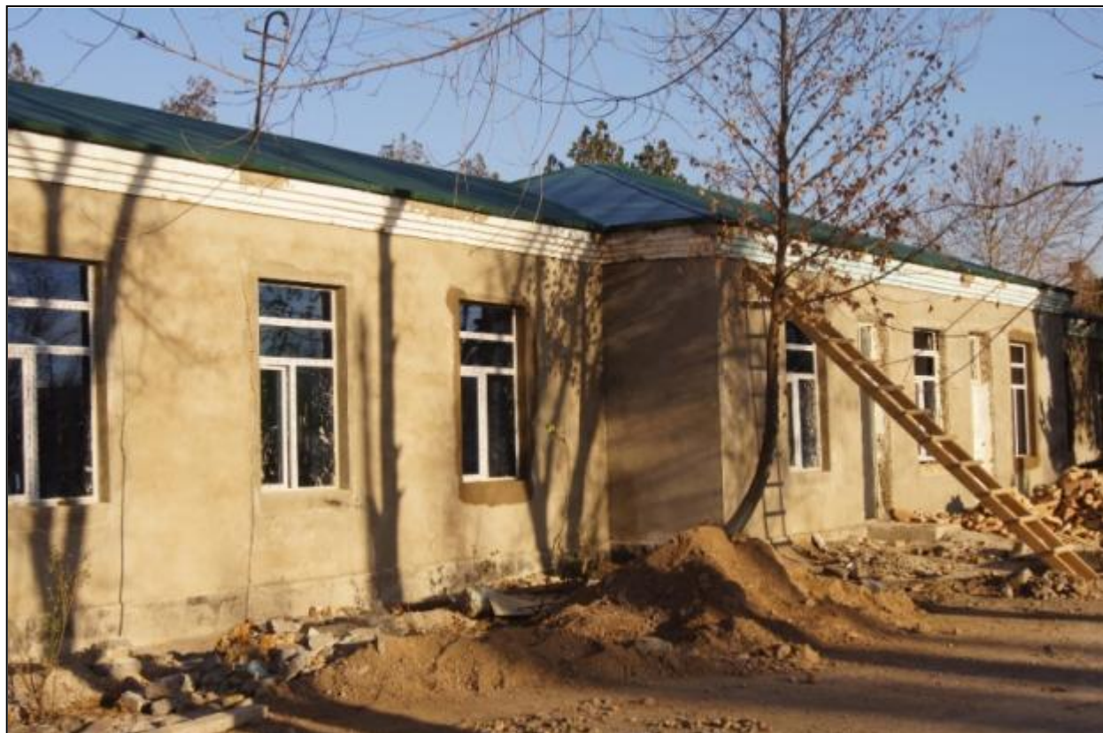
Mastcho Central District Hospital, Mastcho District, Sughd Region, Tajikistan (Photo by UNDP DMRP)
