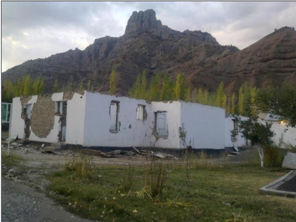
Damaged Tavildara Hospital before Placement of Seismic Beam, Tavildara District, Rasht Valley, Tajikistan (Photo by UNDP DRMP)
