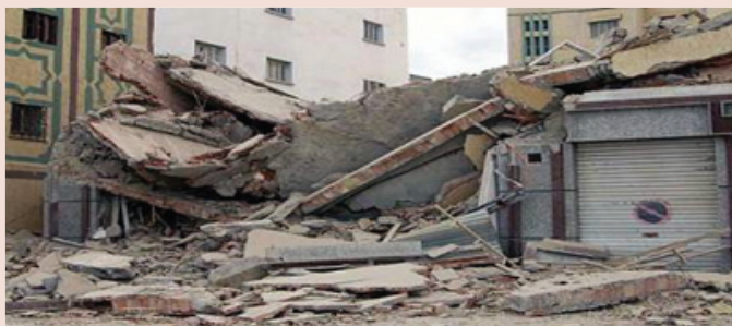
Destruction during Al-Hoceima earthquake, 2004
