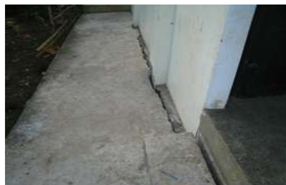
Figure 3.25 A crack at the side of the village hall
