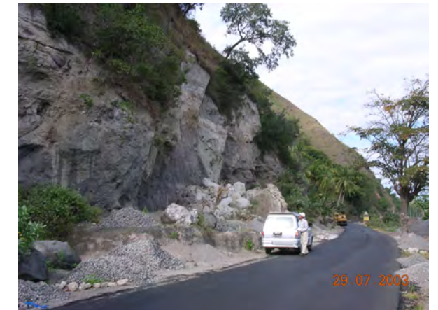
Picture of a rockfall.
