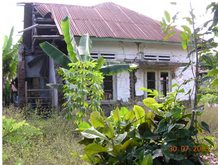
House showing typical earthquake related damages.
