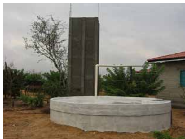
Figure 1: Household Rainwater Cistern Source: REDEH
