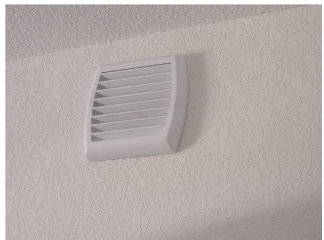
Fig. 2. MVHR vent in an apartment.
