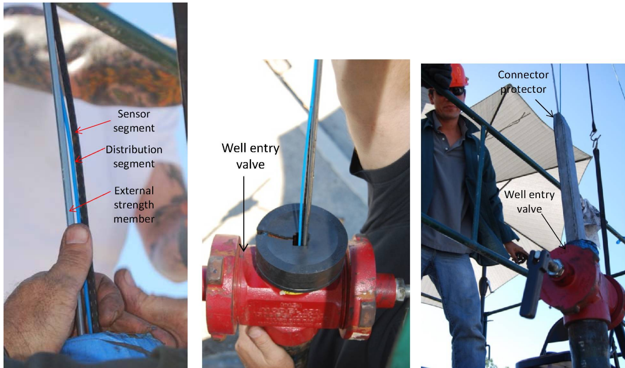
Figure 56 (left and center) Details of the three members that were pulled down together. (right) Introduction of the connector protector through the well head.
